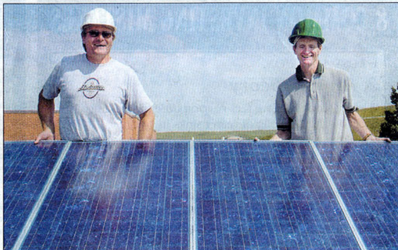
Cochrane High teacher Earl Binder, left, helped install the solar panels on the roof of the school last July, along with Ken Newel, a business development manager with the company Soltek Powersource that distributes the panels. CTimes file photo
